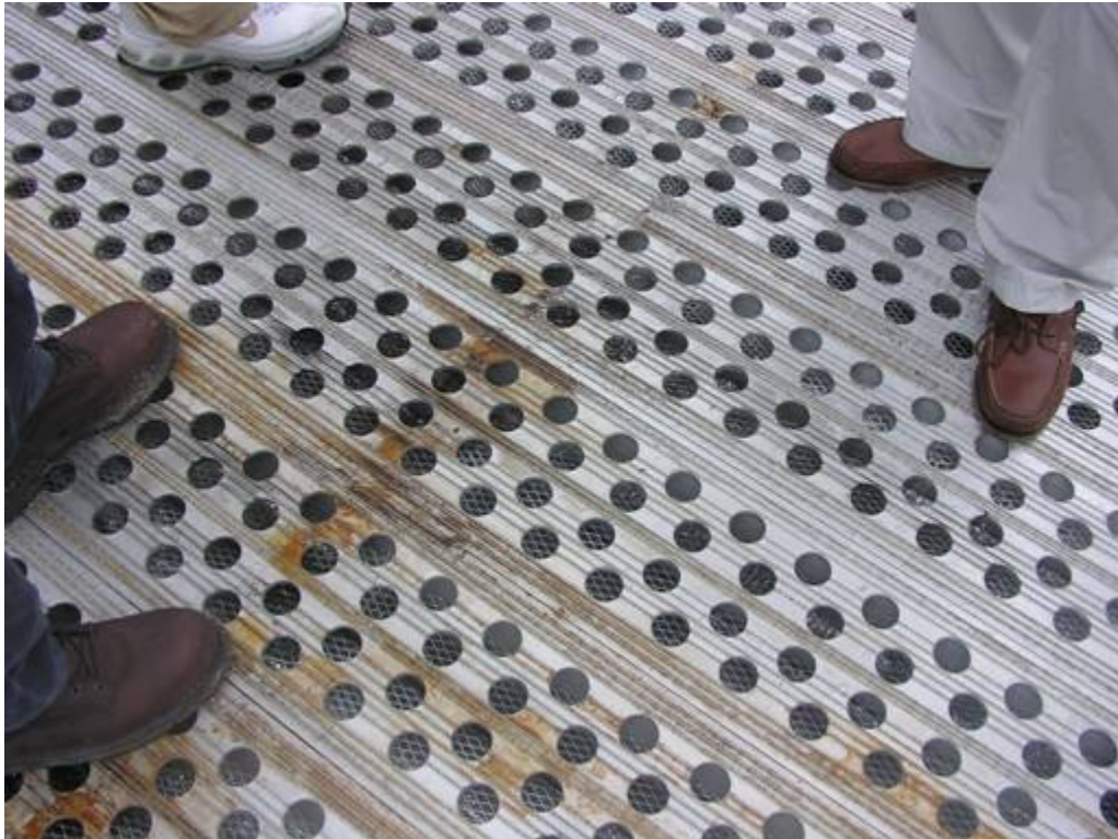
Burning fuel is quickly drained away thru the perforations on the XE Enhanced Safety helideck. This photo is taken moments after a major fire on a safety helideck and you can see from the 'civilian' footwear that the heat from the fire has not heated up the surface appreciably.
